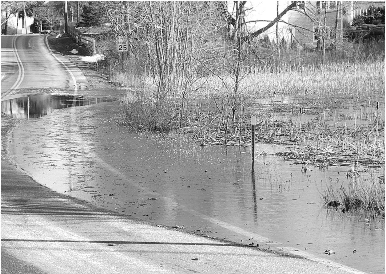
Flooding Wentworth Road at Pit Lane in January 2024. Jim Cerny photo
